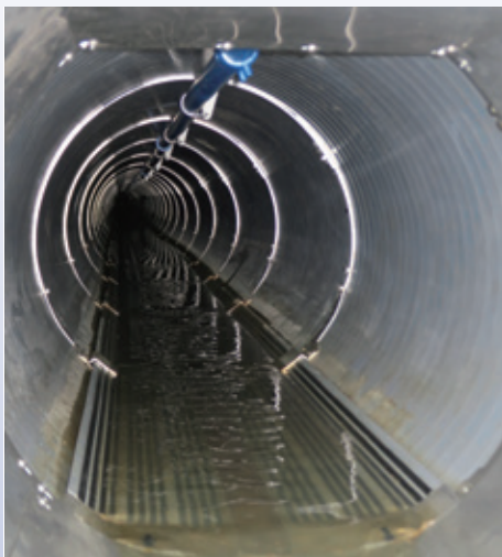
A heat-collecting pipe installed under the surface of sewage in a sewer pipe (black lines)
