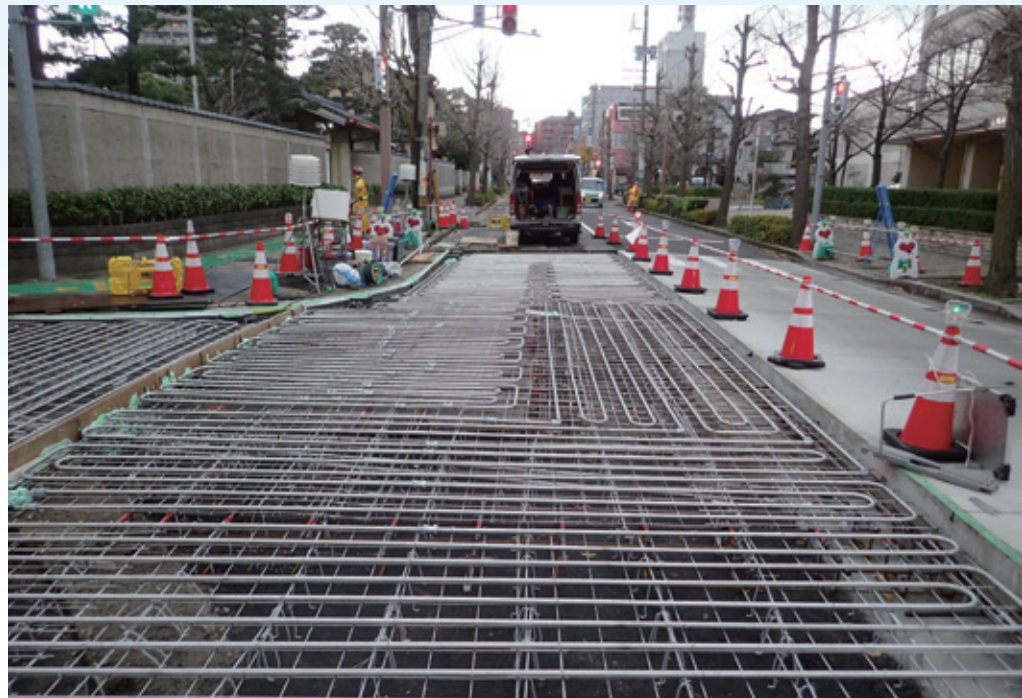
Heat radiation panels installed on a road in Niigata City, Niigata Prefecture for a demonstration test of the sewage heat snow-melting system
