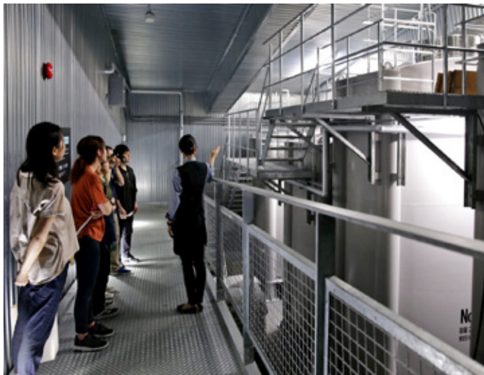
The chill from the snow alone keeps the room temperature at a constant 3 to 4 degrees Celsius
