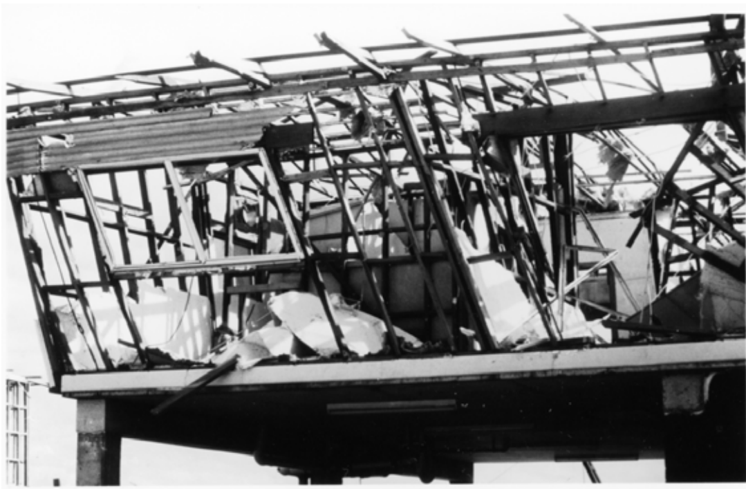
Fig. 5.10 - Failure by racking
