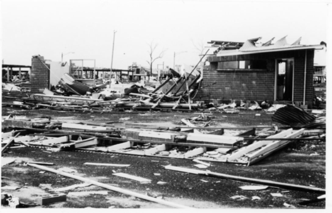
Fig. 5.14 - Failure of recent low set masonry home
