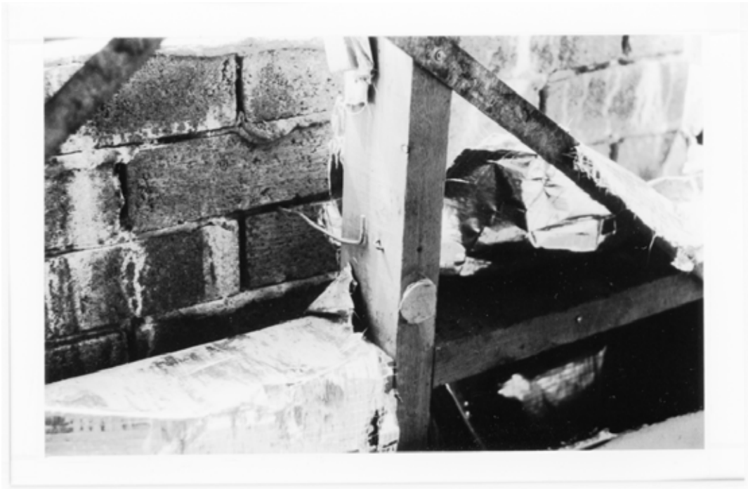
Failure of tie in brick veneer
