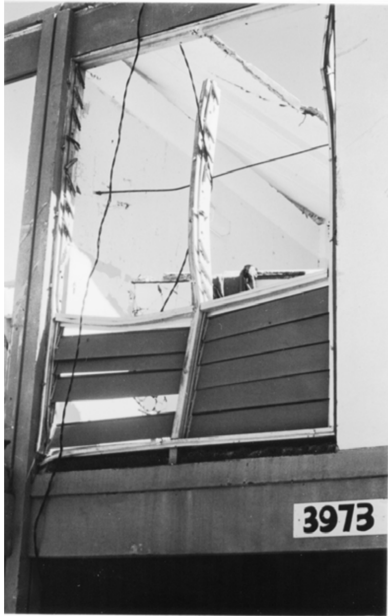
Fig. 5.26 - Battered window frame in concrete house
