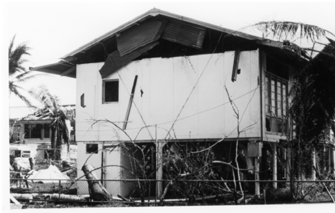
Fig. 6.4 - Damage to windward wall of house in Figure 6.3
