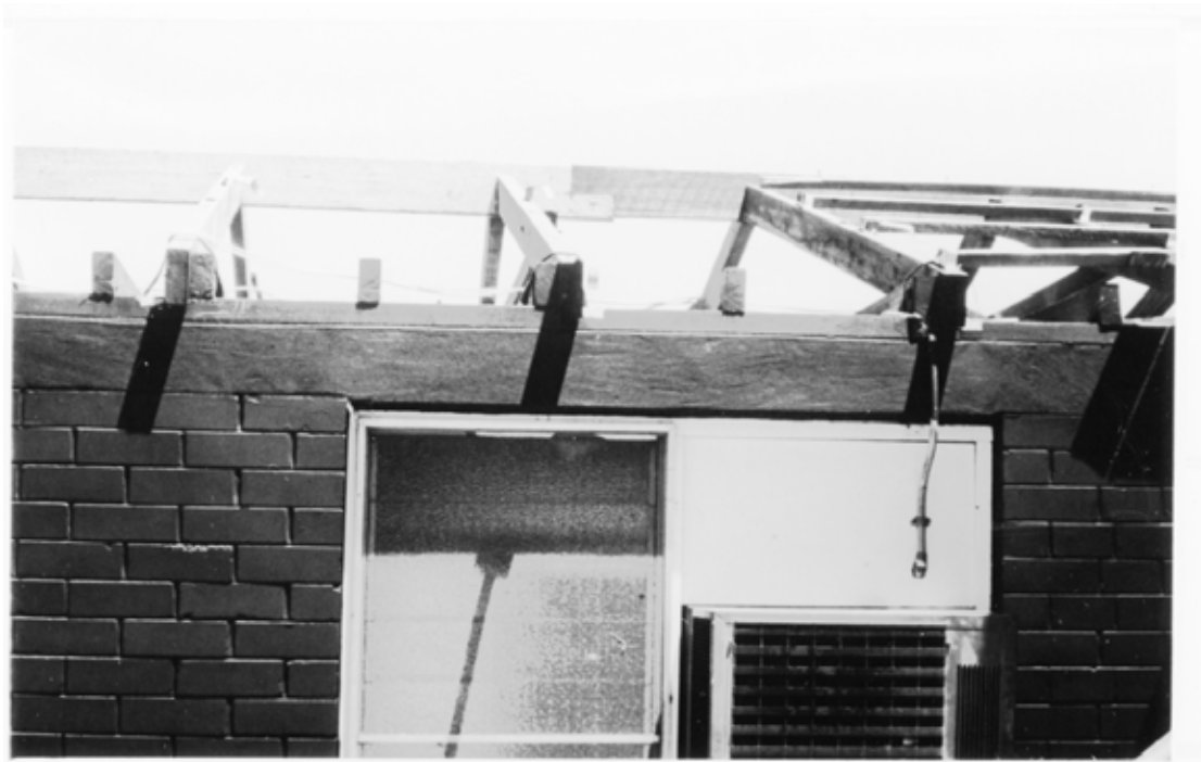
Fig. 5.2 - Roof cladding lost with purlins
