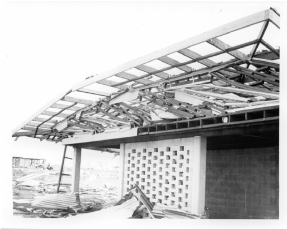
Fig. 512 - Collapse due to racking
