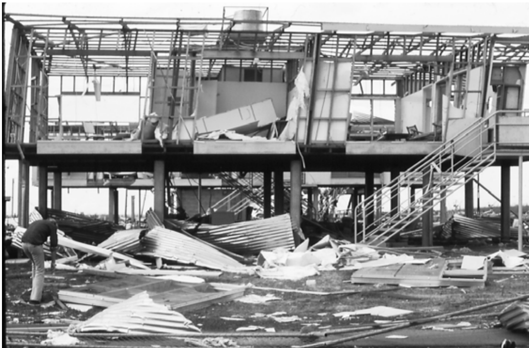
Fig. 5.23 - Having lost wall cladding
