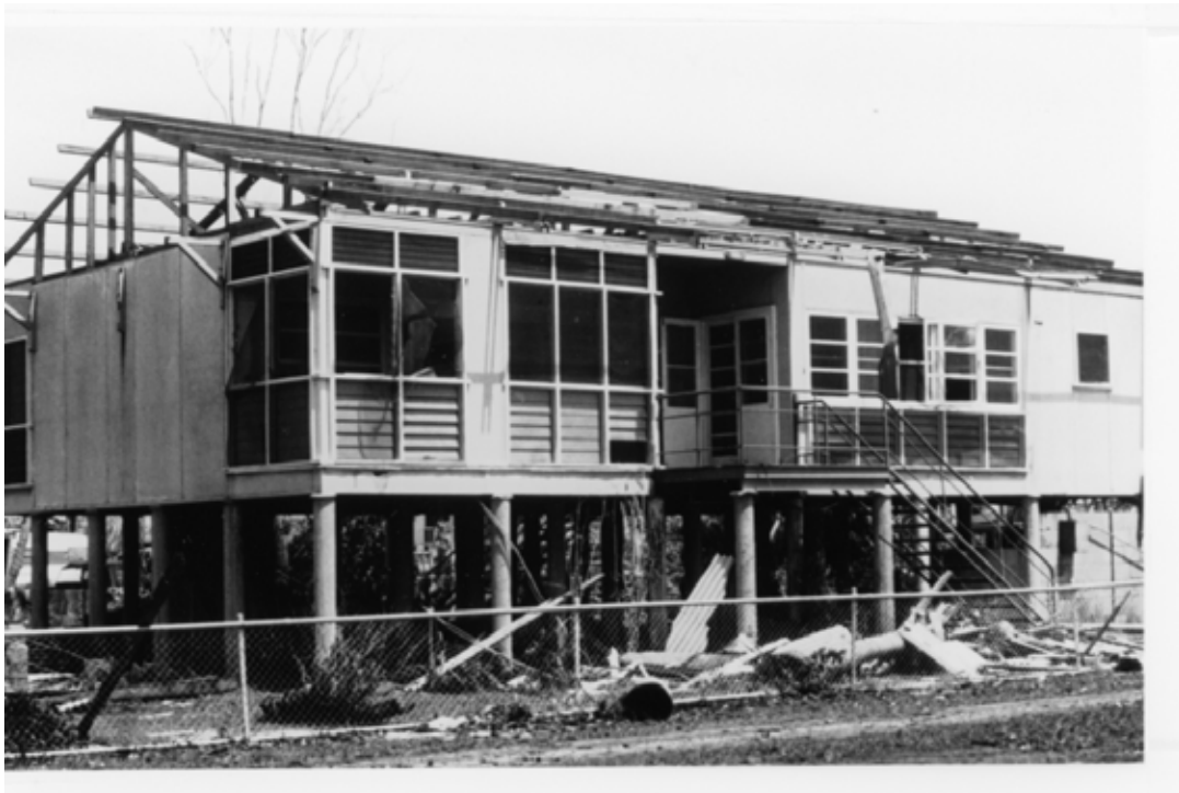
Fig. 5.1 - Roof cladding loss – timber cleated purlins
