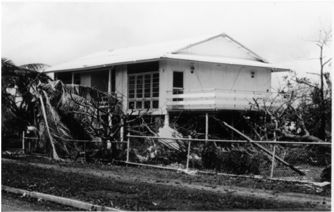
Fig. 6.3 - Performance of house strengthened with battens over the top of the roof
