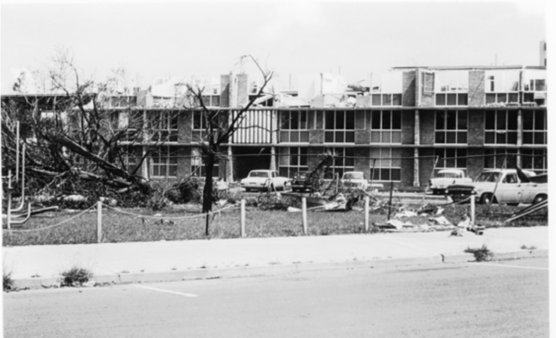
Fig 5.18 - Typical damage to flats
