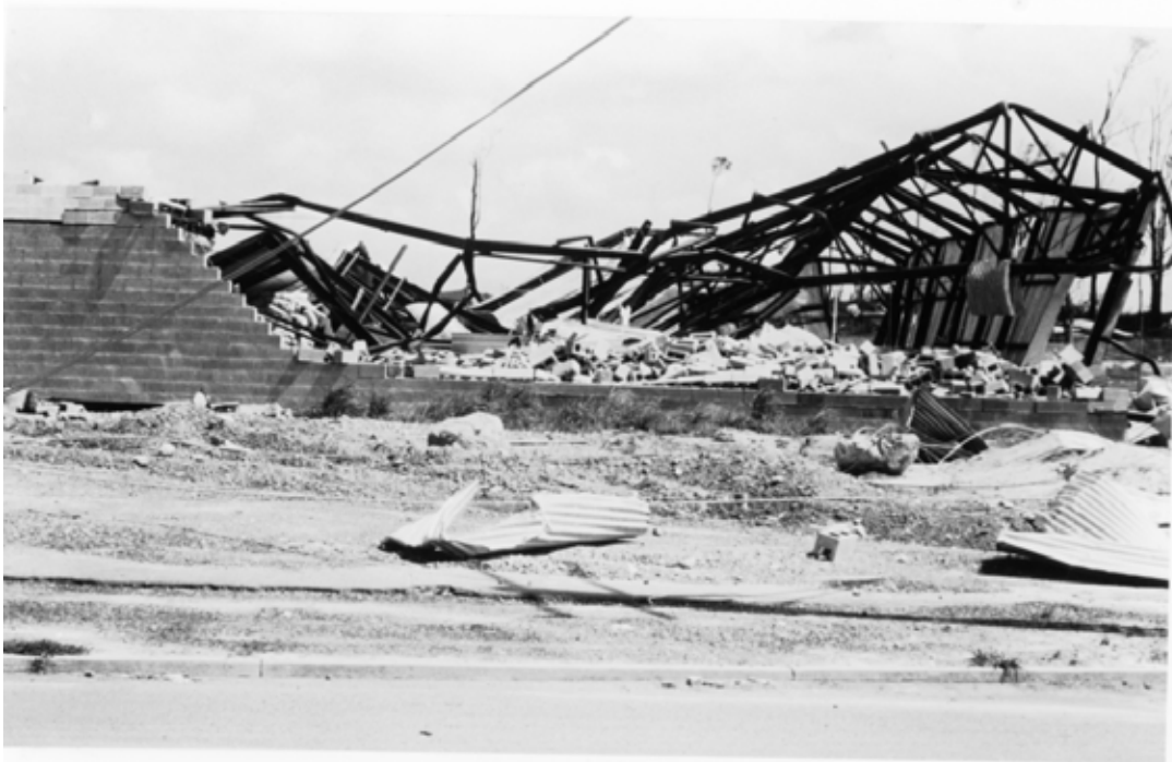
Fig. 5.21 - Collapsed steel building
